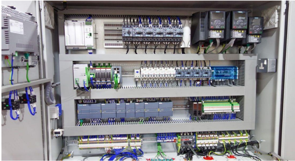
Siemens PLC Panel
