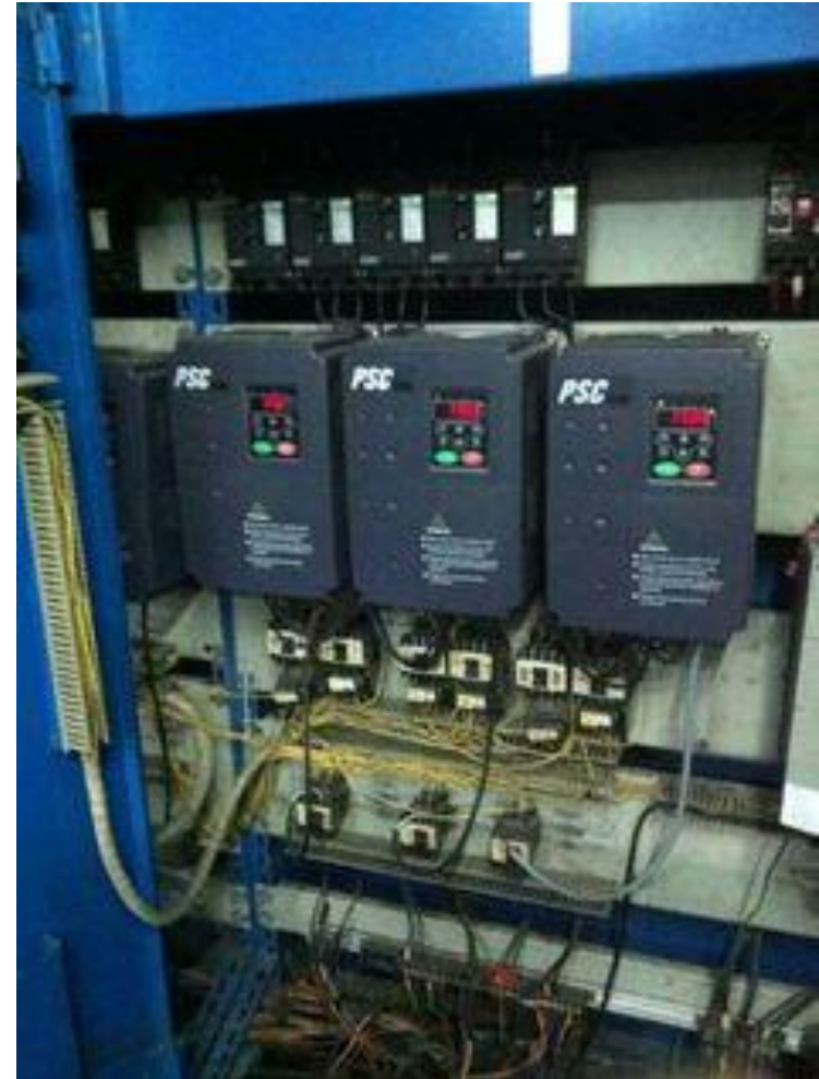
Inverter Control Panel
